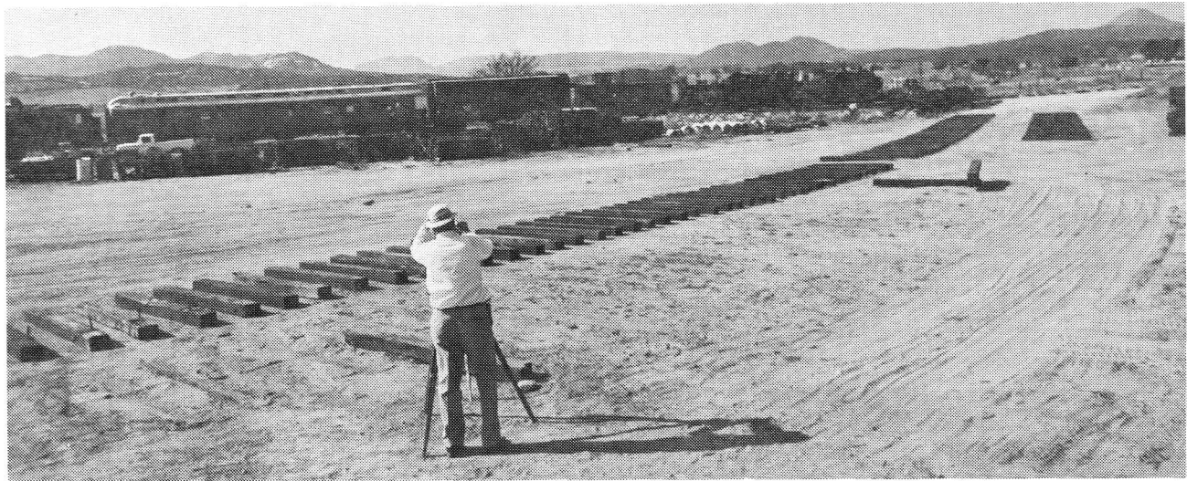
Civil engineer Russ Kimball sights through his transit set up on the point of intersection of the curve on track two. The yard lead switch is just around the bend at right. (Larry Rose photo)
