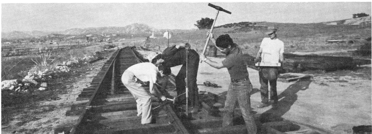
Geoff Shepherd, right, watches three San Diego Trolley operators drive spikes at the PSRM yard throat lead switch. The trolley jockeys from left, are: Larry "Grandma" Granfield, seniority No. 1; Jim Lundquist, seniority No. 2; and Duane Leal, seniority No. 6. (Larry Rose photo)
