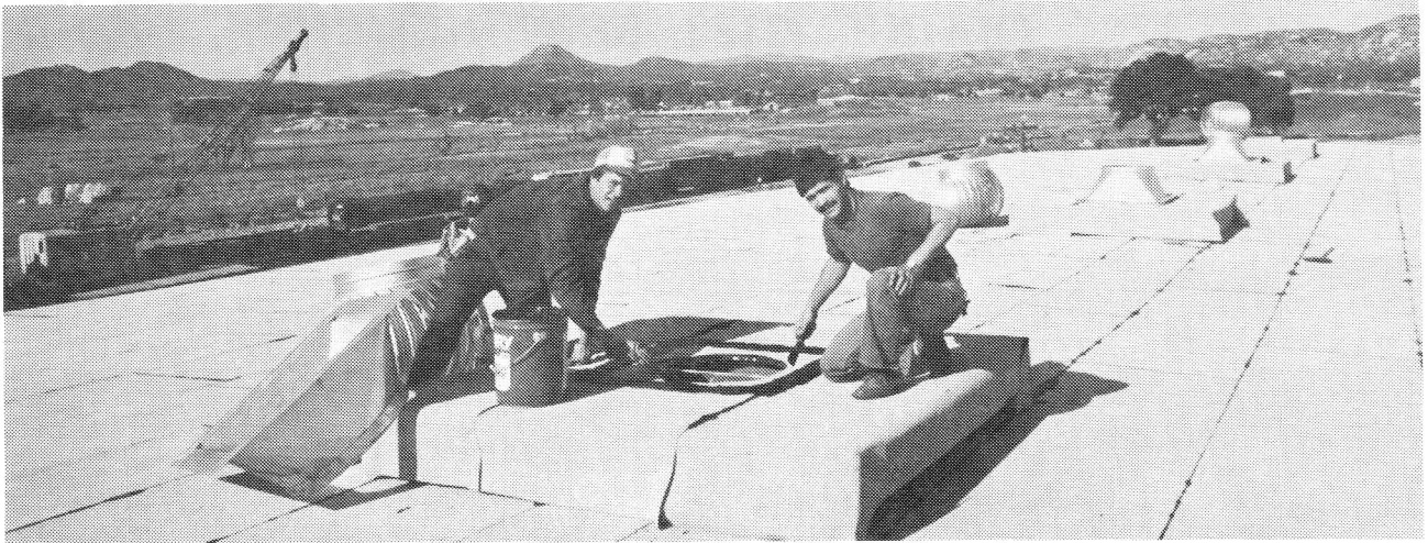
Museum Executive Director Jim Lundquist and member Duane Leal spread mastic in preparation for wind turbine installation on the freshly redone car shop roof. (Larry Rose photo)
